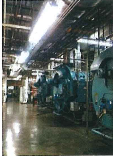
Steam Boiler System
