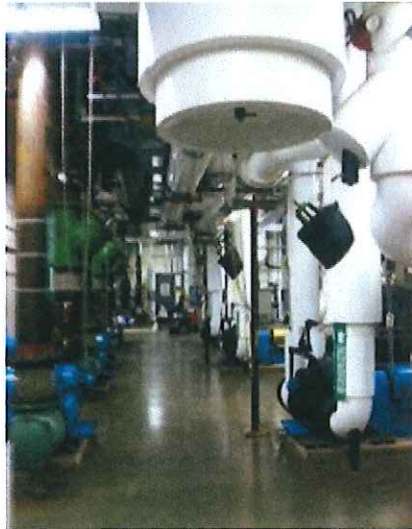
Chilled Water System
