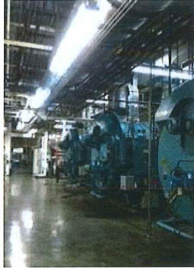
Steam Boiler System
