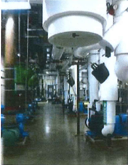
Chilled Water System
