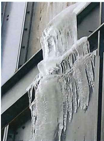
Frozen water penetrated through cooling tower structural beam
