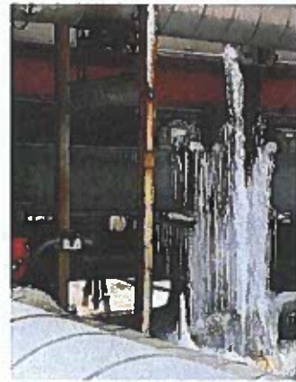
Water and chemicals overflowing cooling tower catch basin onto roof
