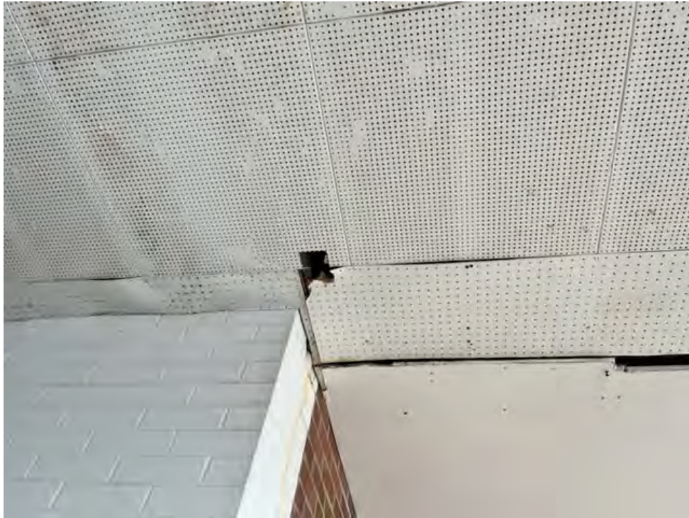
Buildings 1, 2, 3, 4 – representative ACM light grey cementitious perforated panel ceiling of walkway canopy roof
