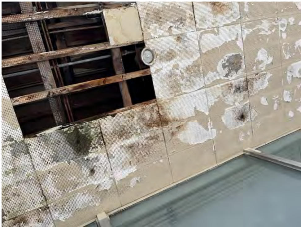
Buildings 1, 2, 3, 4 – representative ACM light grey cementitious perforated panel ceiling of walkway canopy roof
