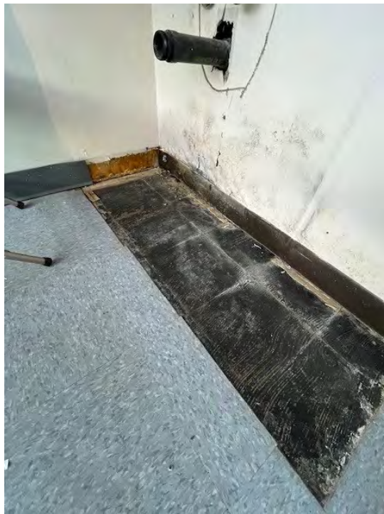
ACM Black original 9"x9" floor tile mastic (throughout buildings floors)
