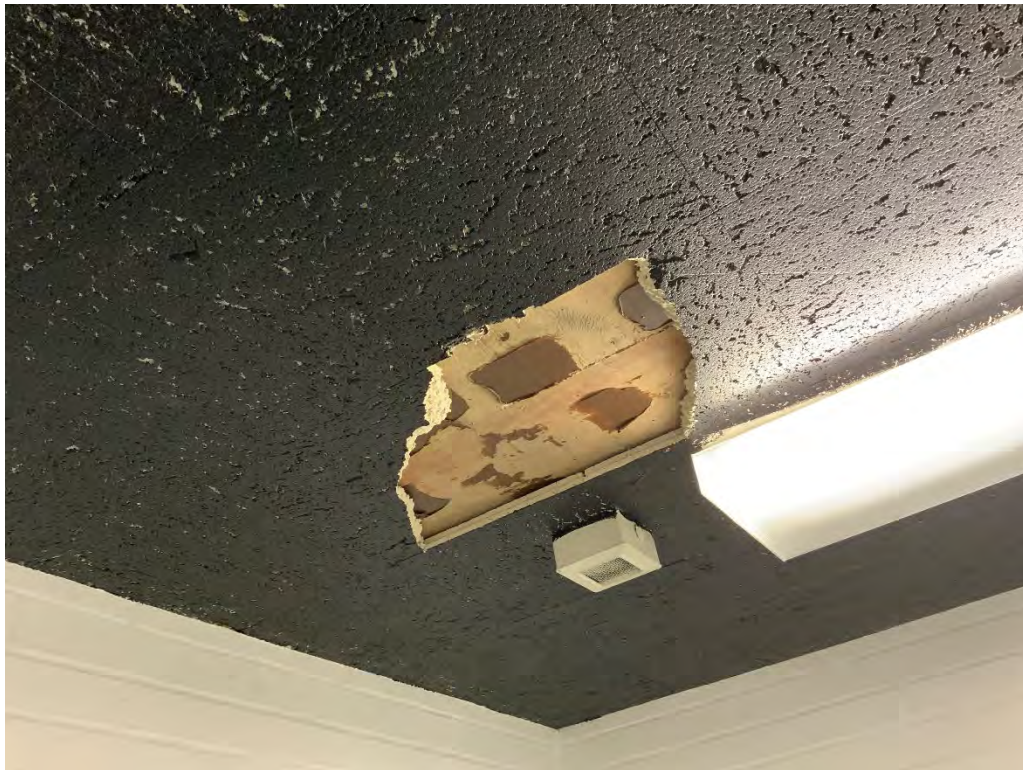
810 Northeast room - ACM Dark brown glue daubs associated with 1'x1' ceiling tiles.
