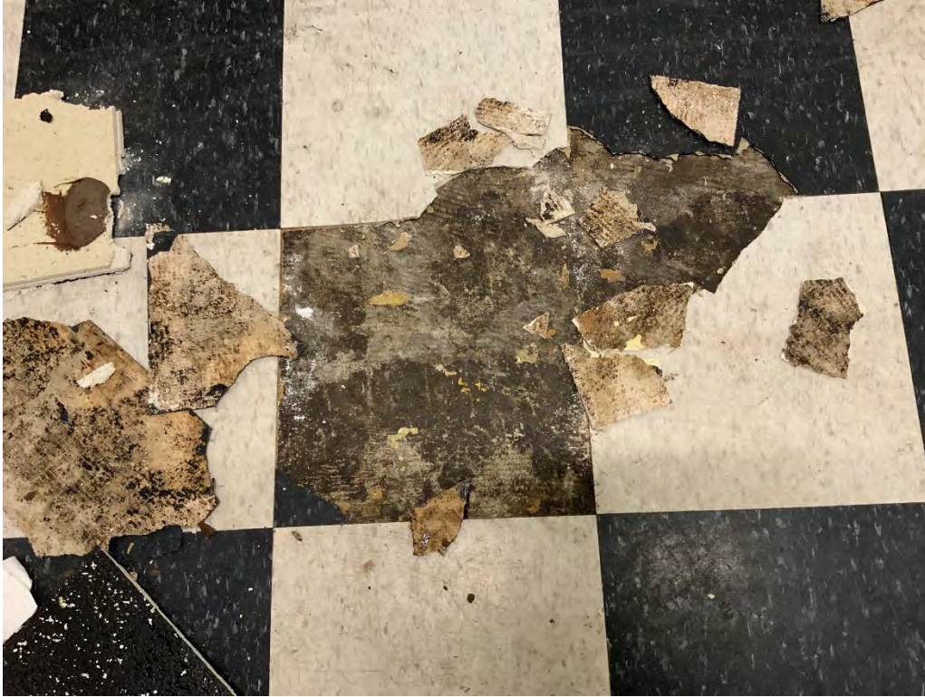
ACM Residual black mastic associated with floor tiles.
