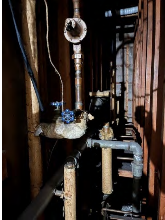
Men's bathroom pipe chase and ACM gray mudded fittings
