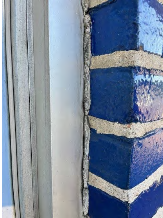
Light grey vertical caulk along exterior wall (multiple areas on single story building)
